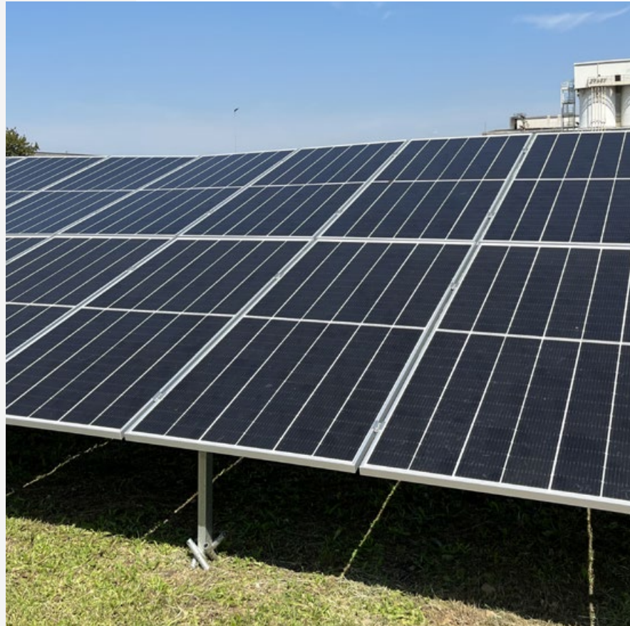
Solar park at Grünenthal's manufacturing site in Origgio
